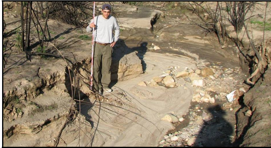
Figure 2.8: Bank failure at Hicks Canyon (Orange County) exhibiting combinations of fluvial erosion, shallow slips, and mass failure in weakly-cohesive, poorly-consolidated banks
