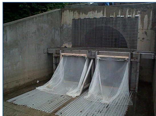
Figure 5. Netting TrashTrap (End-of-Pipe Model)
