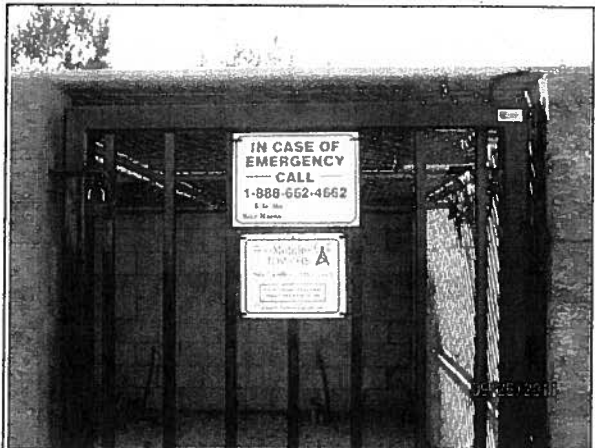
16. Detail of signage on T-Mobile equipment enclosure.
