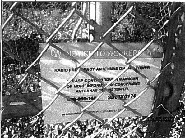
21. Detail of signage on Sprint sector A antennas.
