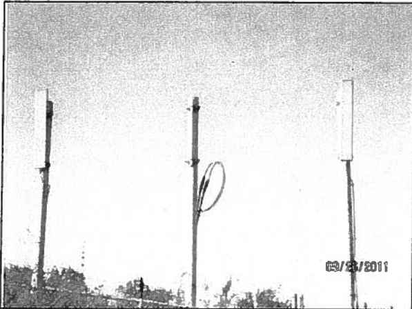
19. View north toward Sprint sector B antennas.
