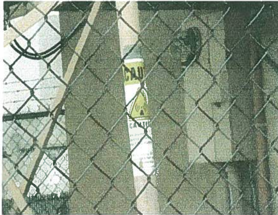
Caution sign at AT&T tower
