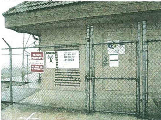
Notice sign on at AT&T fence
