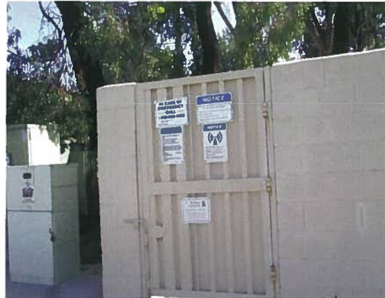
Notice and Info Sign at ATT and T-Mobile BTS
