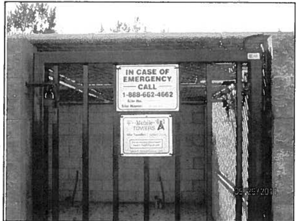
16. Detail of signage on T-Mobile equipment enclosure.
