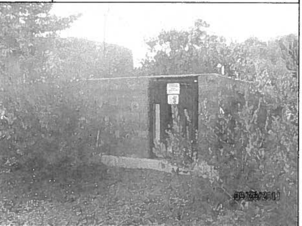
15. View north-northwest toward T-Mobile equipment enclosure.
