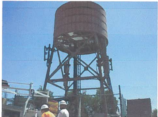
AT&T Sectors A, B & C inside faux water tank (9 total)
