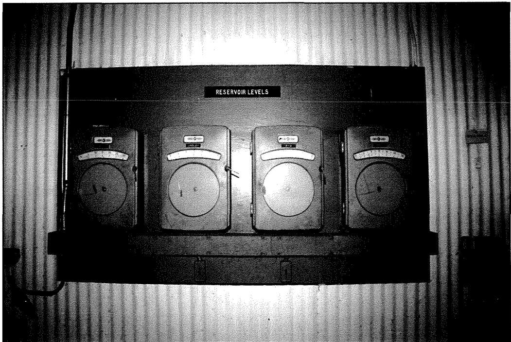
PHOTOGRAPH 20 "Reservoir Levels" Panel on Side of Northern Office
