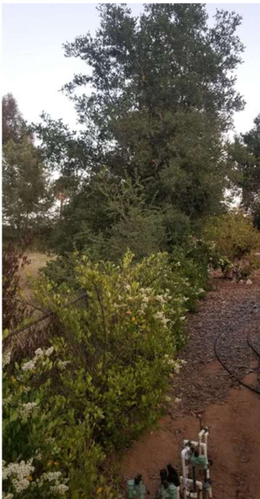
Figure 3c – Example of tree/shrub growth through the property line fence and proximity of sprinkler set to fence.
