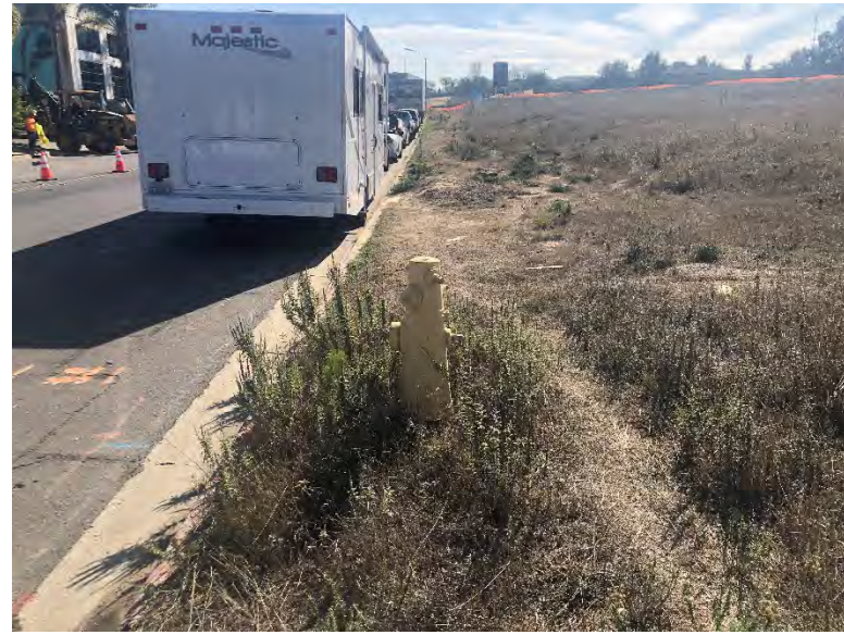
Photo 14: Myers easement fire water utility
