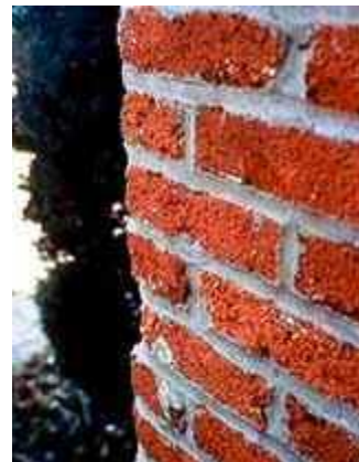
DAMAGED SANDBLASTED MASONRY
