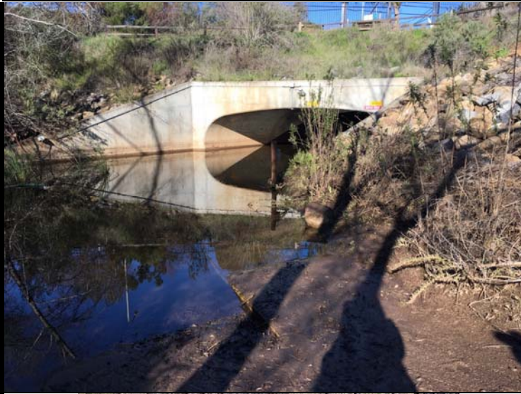
Representative Photograph 1. Facing NW. Large box culvert outlet at upstream portion of channel.
