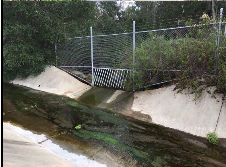
Representative Photograph 2. Facing S. Inlet for adjacent natural channel flowing into concrete-lined channel.
