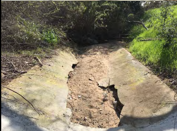
Representative Photograph 3. Facing NW. Portions of concrete is broken and in need of repairs.
