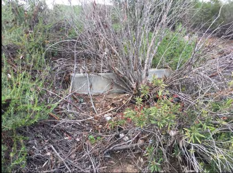
Representative Photograph 2. Facing E. Blocked outfall
