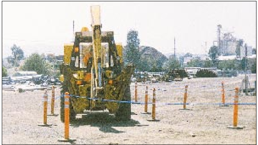
Obstacle Course. Backhoe operators must demonstrate the ability to maneuver forward and backward through a delineated course.
